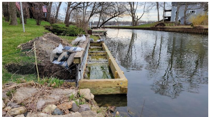
Photo 4. Shoreline project with exposed sediment piles, excavated soils, construction debris which impact overall channel and lake health.
