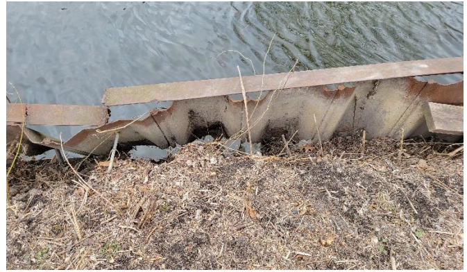
Photo 6. Seawalls no longer offer shoreline protection.
