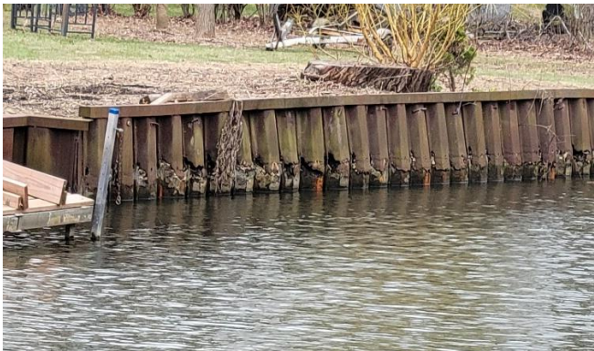
Photo 3. Example of failing seawall on the channel.
